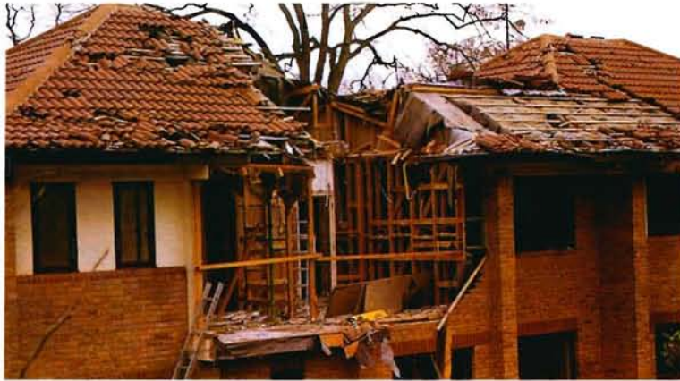
Mr Smith's home with its roof missing
