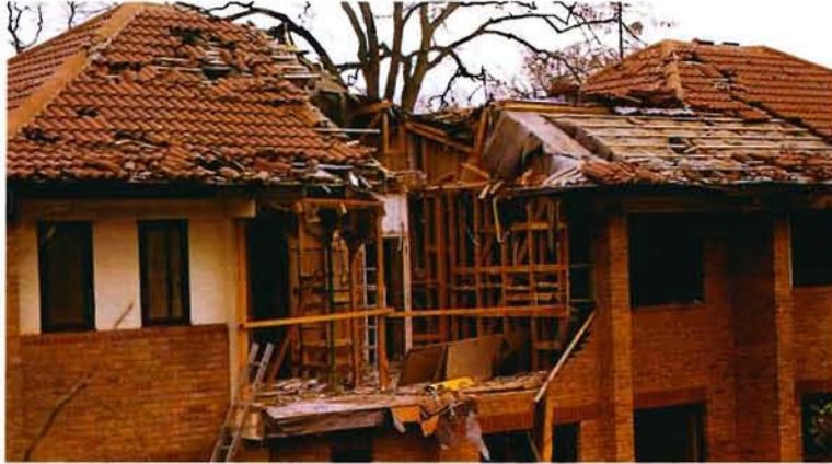
Mr Smith's home with its roof missing
